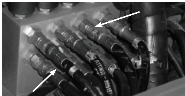
Figure 7.14 - Check Fittings at Valve
