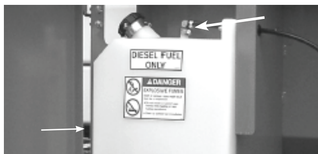
Figure 7.3 - Fuel Leaks at Tank
