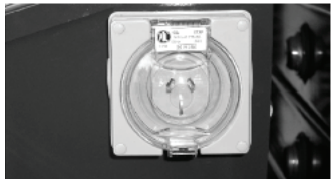
Figure 11.7 - Mains Power Connection For Charger
